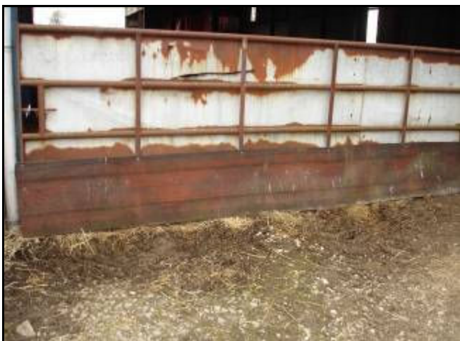
Fig 9: Gaps under gates must not be able to be enlarged by digging.
